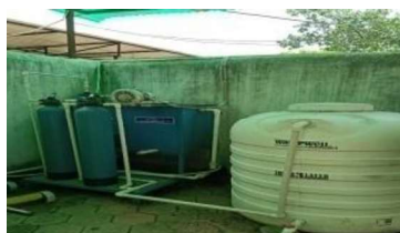
ETP Plant unit
