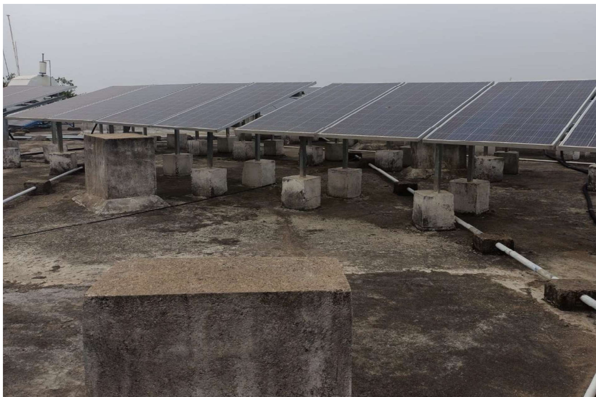
Fig-11: A unit of solar Panel
